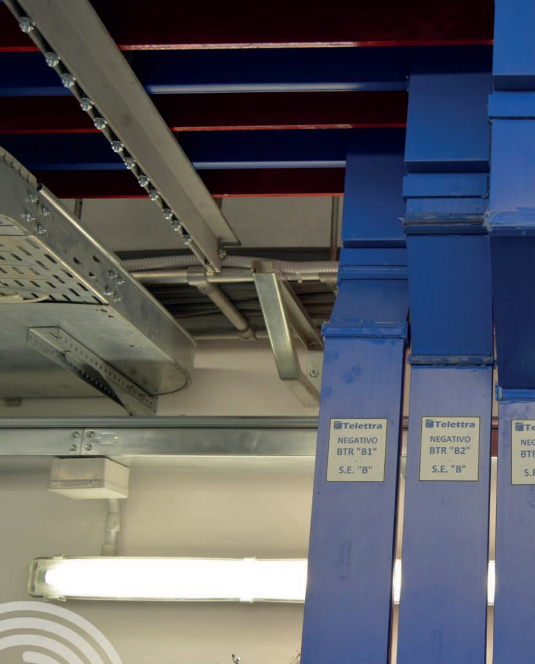
Collegamenti corrente continua DC (direct current) connection or cables
